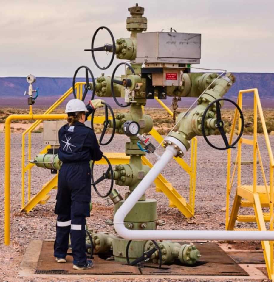
Pictured above: gas lift installation in Aguada Federal block
